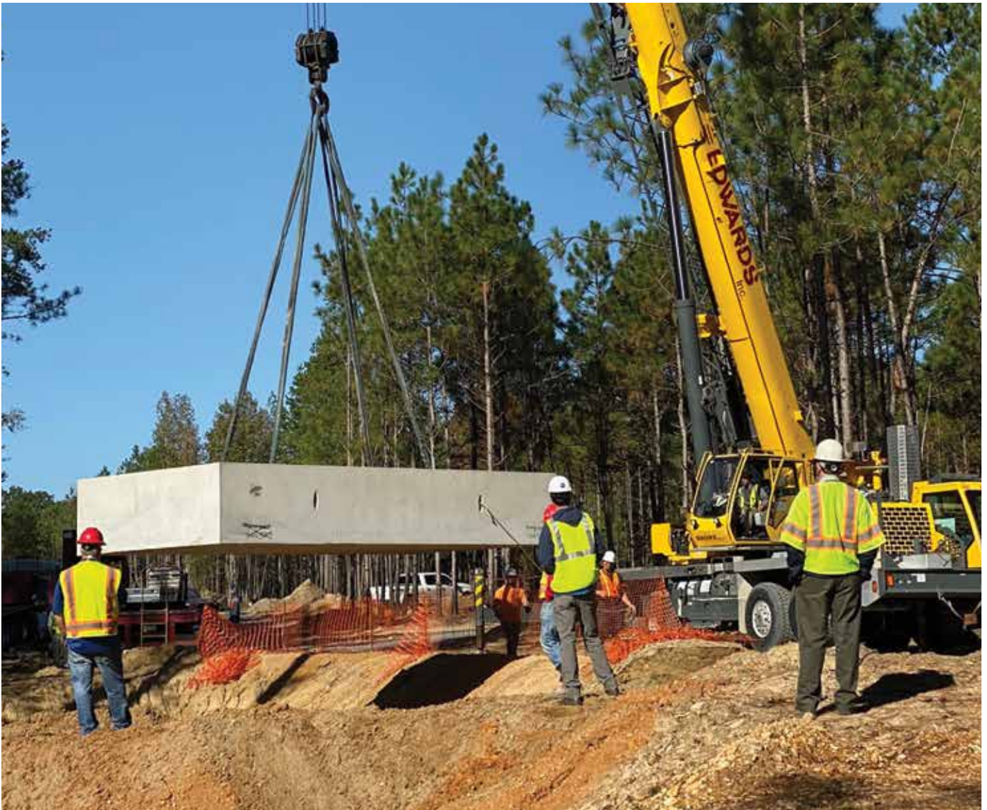
It took just shy of four hours to assemble the tanks with the help of a 110-ton crane.
