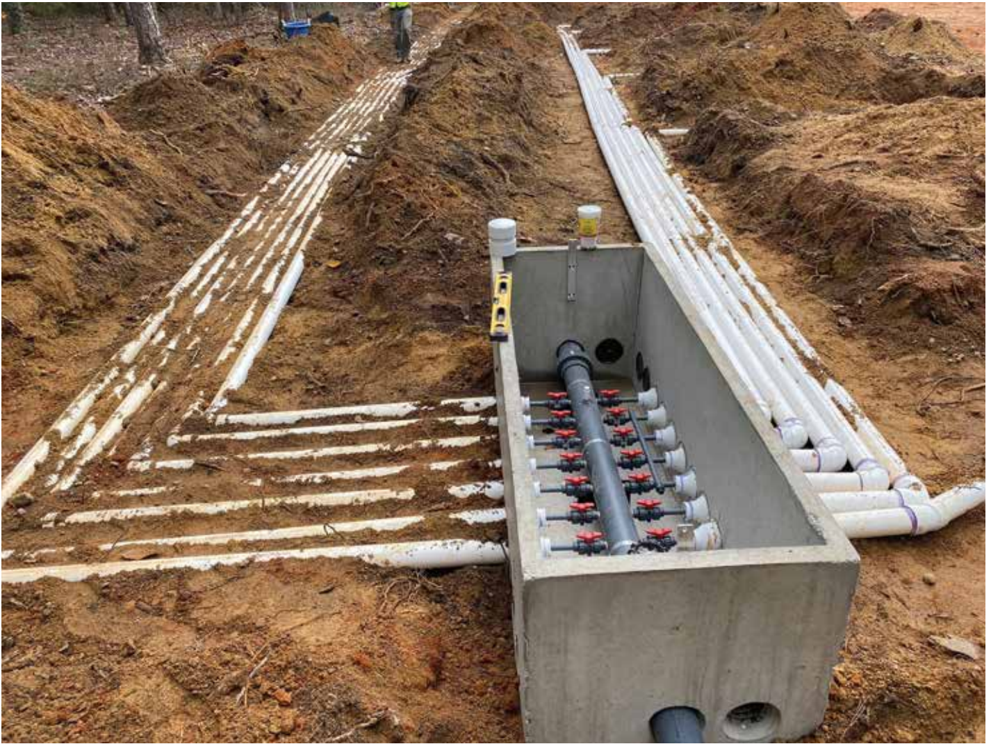
The septic system at Raven Rock State Park was the largest project to date for Shoaf Precast and Creech Plumbing.
