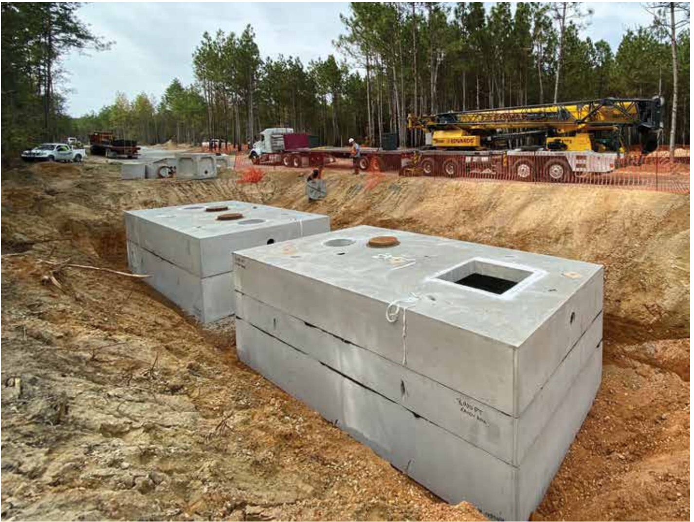
Shoaf Precast manufactured the precast portions of the septic system for the Moccasin Branch campground at Raven Rock State Park in North Carolina.
