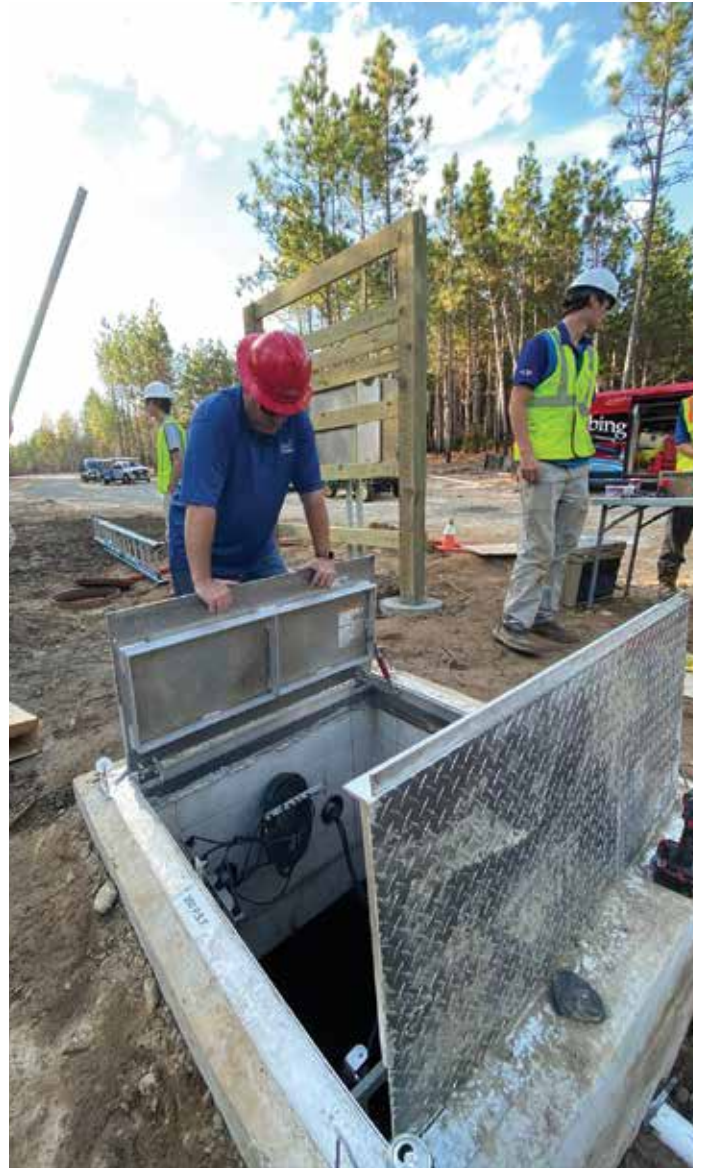
The logistics of the state park project required extensive planning for transport and staging.
